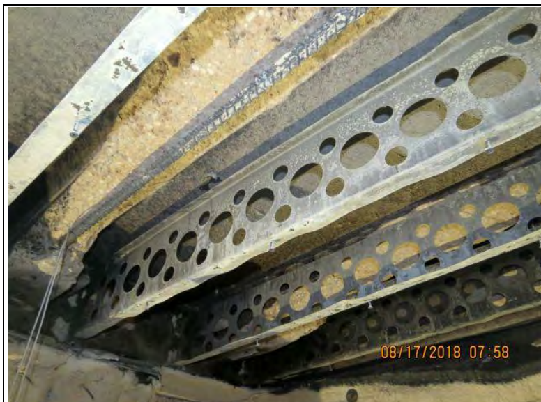
Photo No. 42 Post-test
