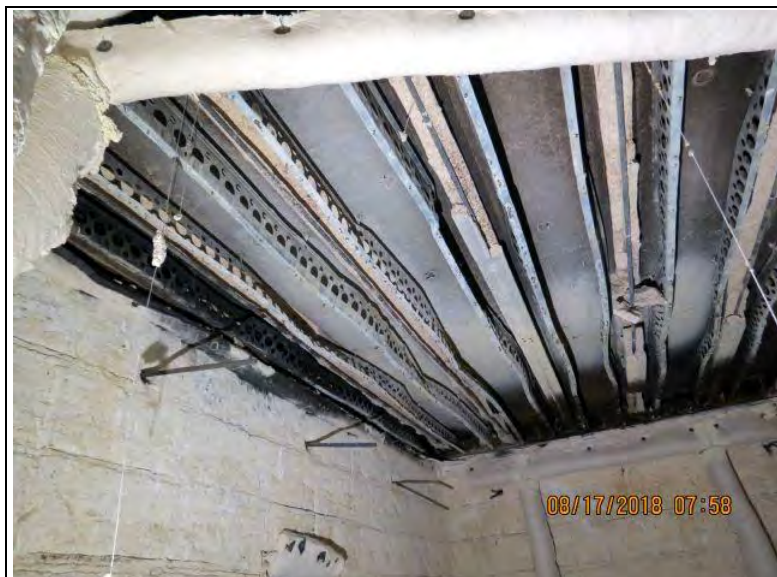
Photo No. 40 Post-test
