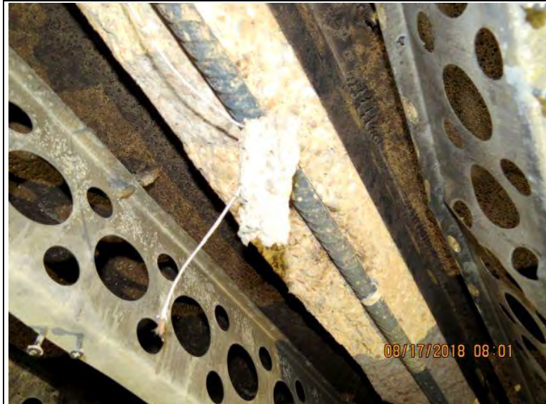
Photo No. 47 Post-test
