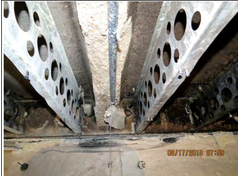
Photo No. 43 Post-test
