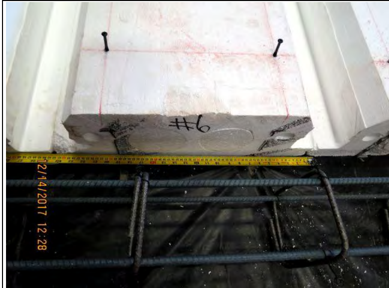
Photo No. 5 Panel width
