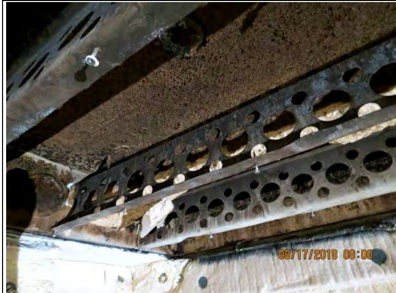
Photo No. 45 Post-test
