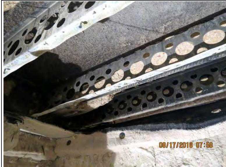
Photo No. 41 Post-test
