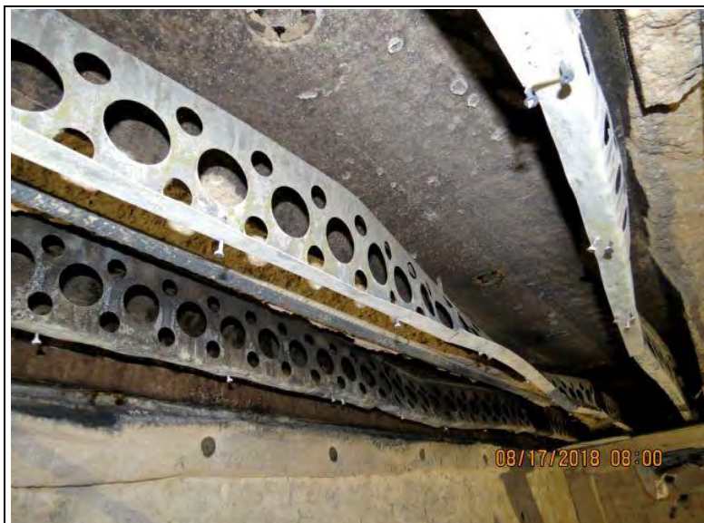
Photo No. 46 Post-test
