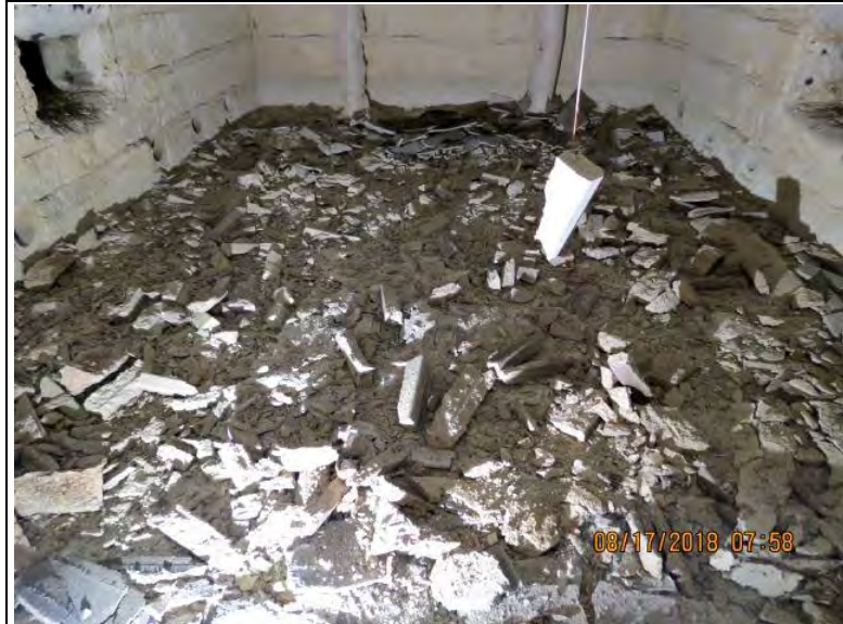
Photo No. 39 Post-test
