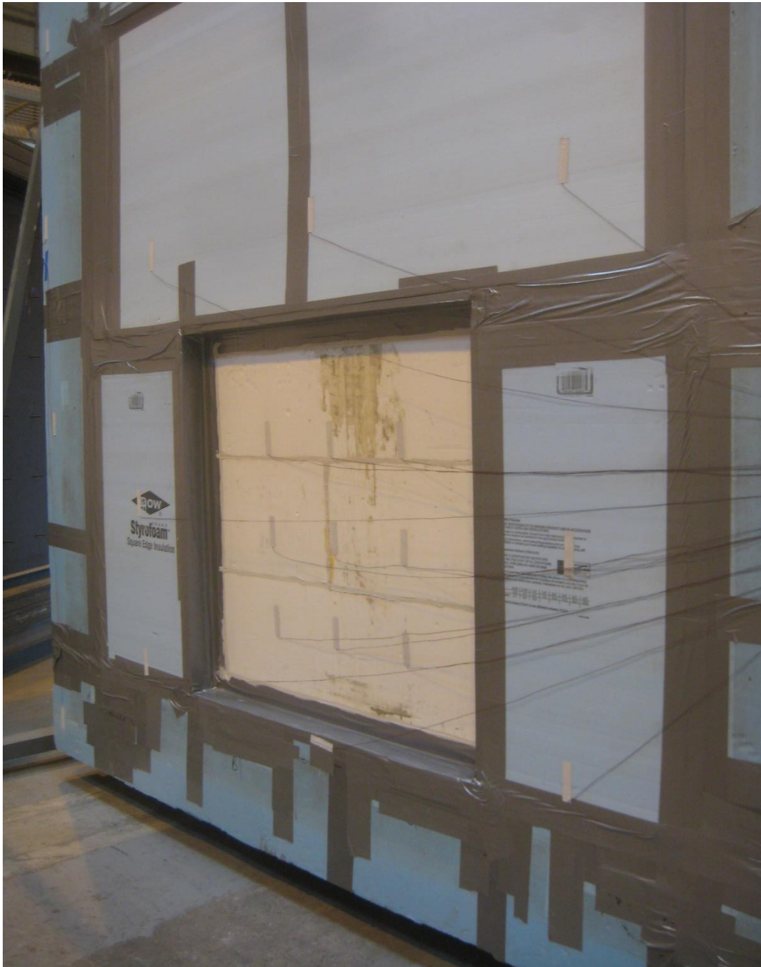
Photo #2, interior of unit installed
