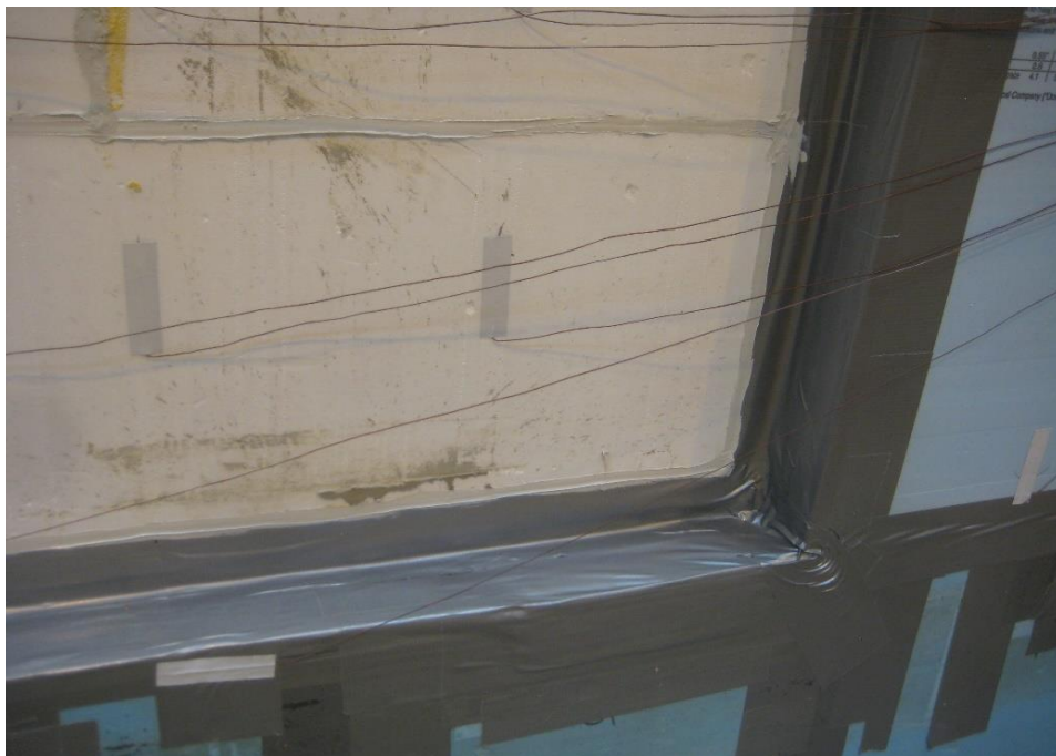
Photo #9, interior of test unit intalled and sealed with duct tape and caulke
